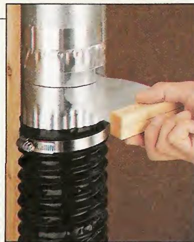
Sliding a shop-made blast gate in and out of a pipe turns the suction off (or on) at each tool.
