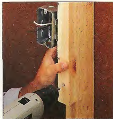
▲ Stud Extension. Extend electrical fixtures so they're flush with your new wall by widening studs with scrap "two-by" material.
