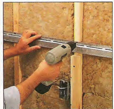
Step 3. With the sound blanket in place, screw lengths of resilient channel to the studs or joists.
