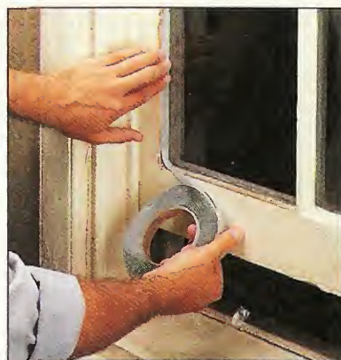
▲ Repair Windows. To seal windows for noise, first replace any broken glass and repair cracked or missing window glazing.
