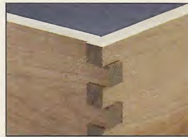
Long Pins. Pins extending well beyond the sides are caused by a router bit that's set too deep.
