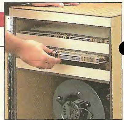
Filters. Ordinary furnace filters above and below the motor/blower clean dust particles out of the air.
