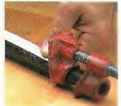
Applying a strip of masking tape to the pipe prevents the iron from reacting with the water in the glue and staining the wood.
