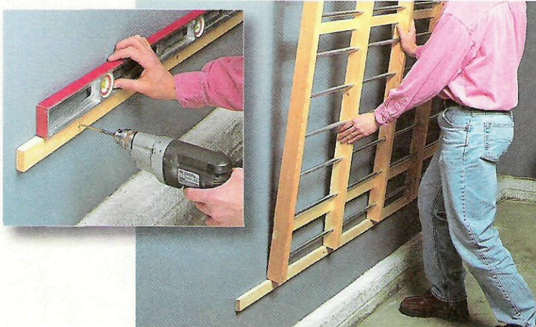
1 A long strip of wood that's temporarily screwed to the wall provides a convenient support as you raise the grid. Just be sure it's level, see inset.
