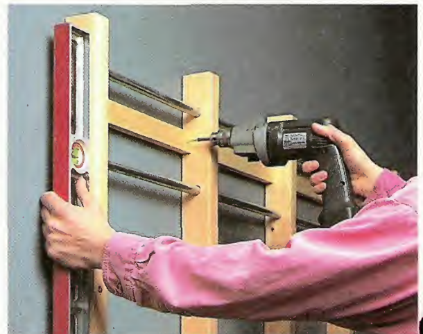
2 After checking that the uprights are level and plumb, attach the grid by driving screws through the cleats and into the wall studs.
