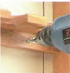
▲ The rack is held securely in place by driving screws through a cleat and into the wall.
