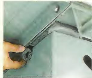
▲ To seal the upper part of the cabinet, stuff in short pieces of foam insulation between the "ribs" of the cast iron table.
