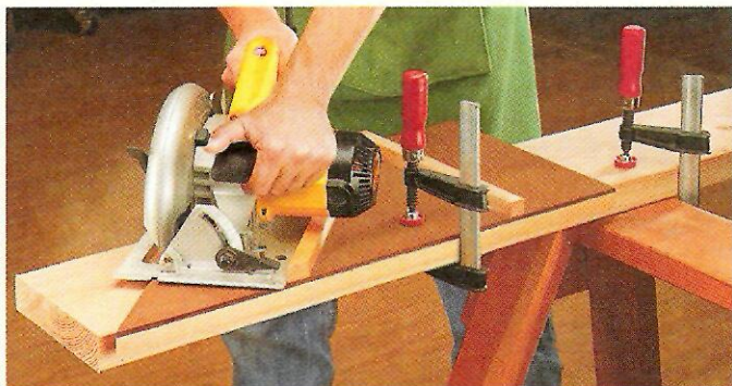
▲ 45° Miters. To make precision 45° miters, align the angled end of the crosscut guide with the layout mark. Then run the base of the saw against the fence as you make a cut.
