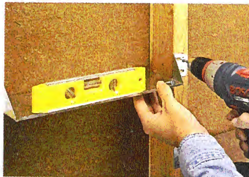
▲ Leveling it Up. Though not required, using a level when installing a shelf makes the task quick, easy, and accurate.
