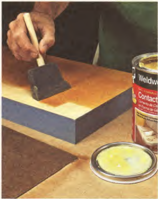
▲ Apply Glue. For best adhesion, apply two coats of contact cement to the laminate and the substrate.
