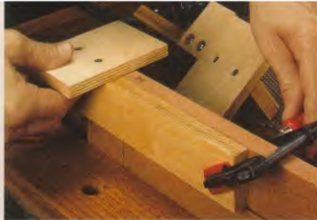
▲ Jig Setup. After marking the location of the hinge on the door, you can position one guide on the mark and clamp it in place.
